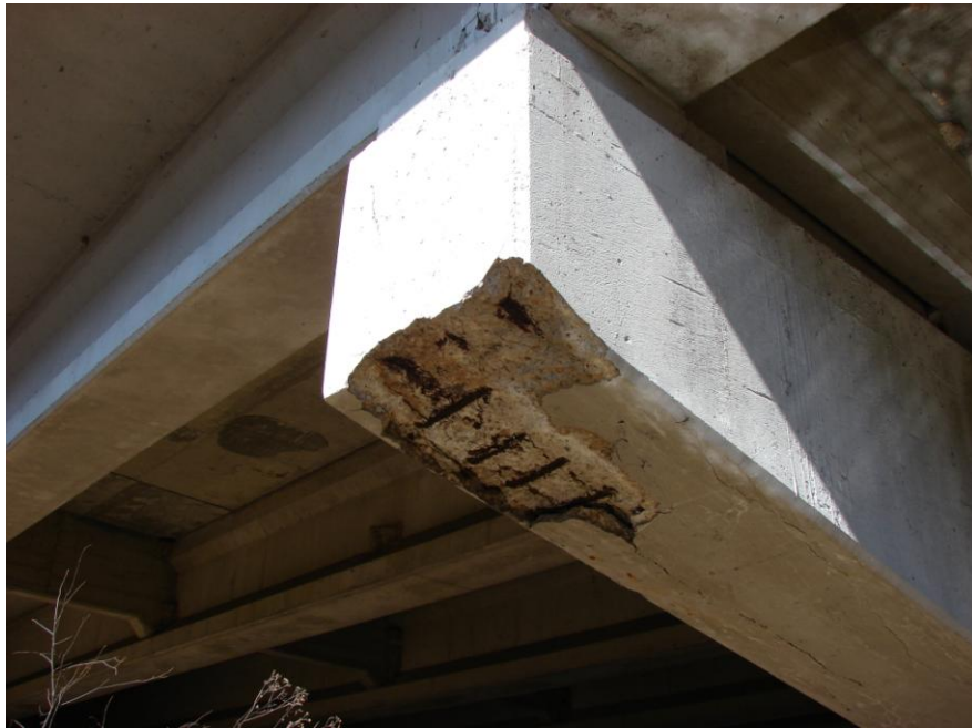
SPALL W/EXP REBAR @ BOTTOM OF CAP R.S. BENT-1
