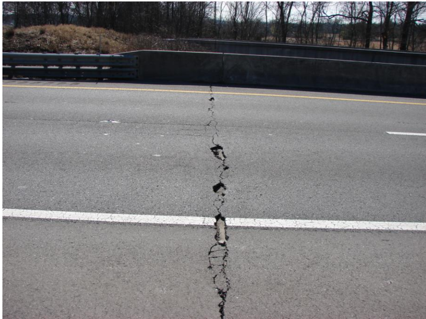
POTHOLES @ B-APPROACH JOINT
